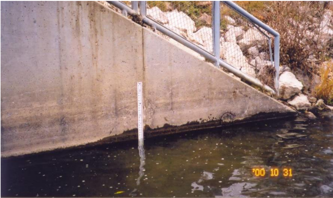
Figure 6-7. An example of a staff gauge installation. Little Goose Creek site LG1 staff gauge (shown above) was secured to the concrete lined channel near the Big Goose Creek confluence.
