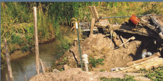
Headgates and diversions in need of rehabilitation would be addressed in the study.
